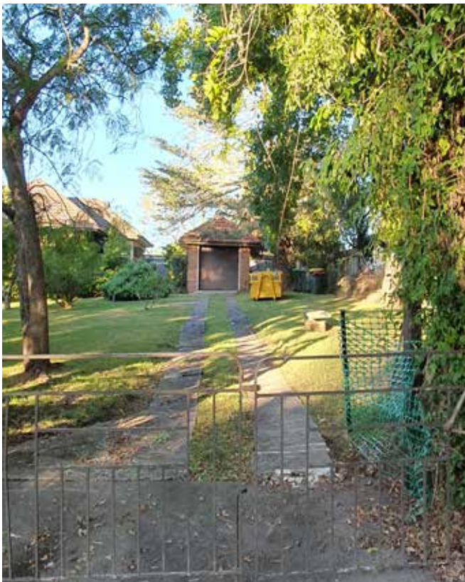
Driveway entry off Hillcrest Road showing poor condition of concrete drive ( Image author May 2021)
