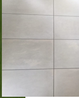
Light grey expressed joint fibre-cement sheet cladding eg. CSR Baresone FC Sheet product, or similar.
