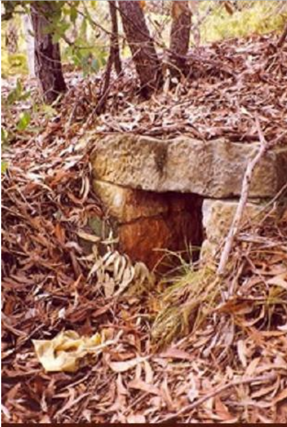
Culvert opening on the outer face of the road, located behind the fence on the roadway.
