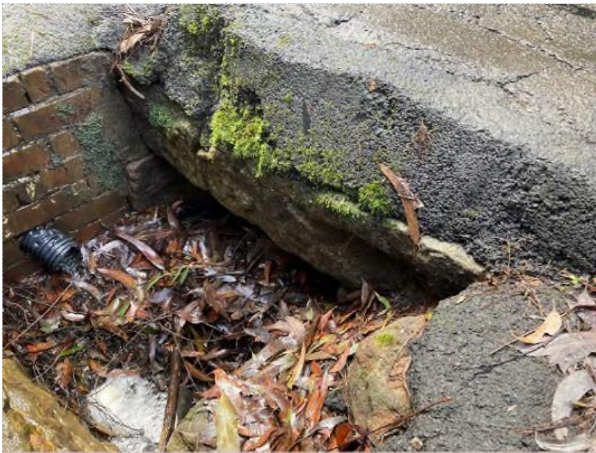
Culvert opening on the inner side of the road relined with brick with some exposed sandstone.
