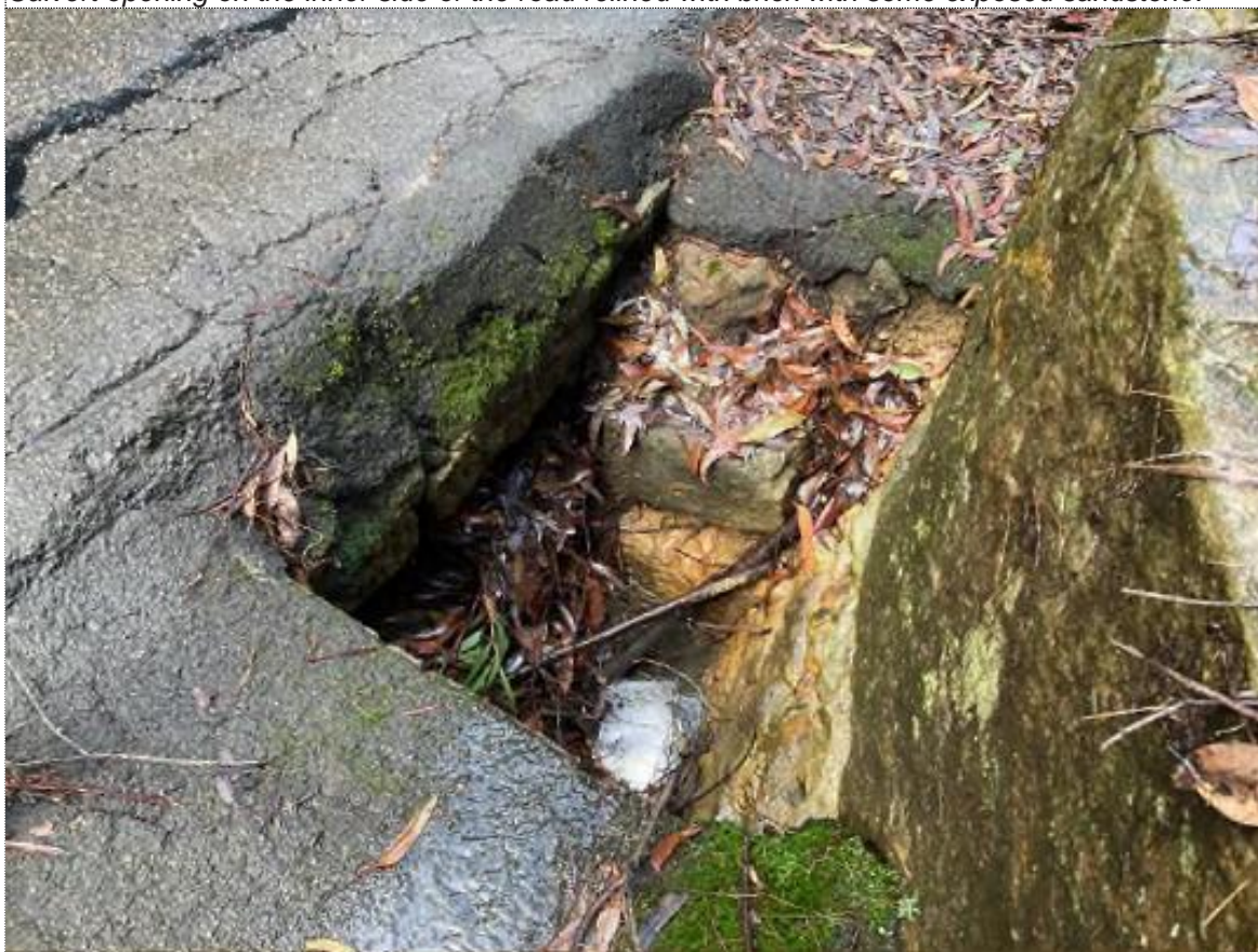
Culvert opening on the inner side of the road with some exposed sandstone.
