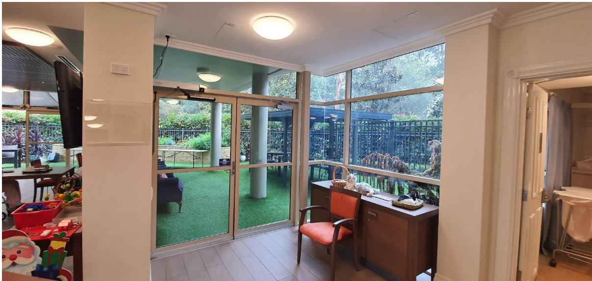
Photo 8: Door to be relocated from inside - note not a required exit.
